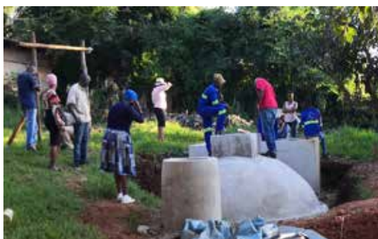
Image 22: An 18m 3 Biogas digester built by Vatsakeme NPO under the UNIVEN-SANEDI partnership to support an emerging farmer with domestic and agro-processing functions in Chavani.
