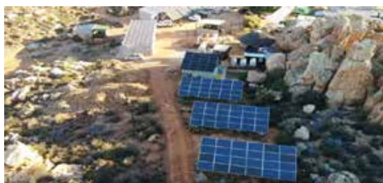
Image 13: An aerial view of the commercial rural pilot test site: Kagga Kamma Nature Reserve in the Cederberg, Western Cape, with the Solar PV and the diesel Gensets in view.
