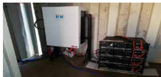
Image 14: PowerStar3/Nomad connected to Pylontec Lithium Ion Rack. The battery and the inverter communicate on the integrated CAN bus.
