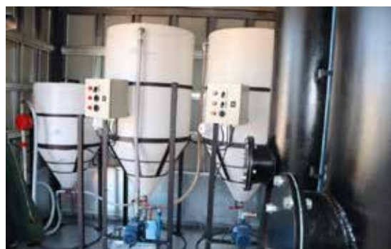
Image 17: Mobile Waste Oil to Biodiesel Processing Plant-Interior
